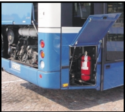
Image 3 - Firetrace system installation.
