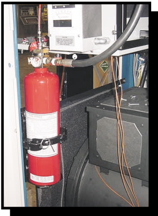
Image 2 - Firetrace system and discharge line
