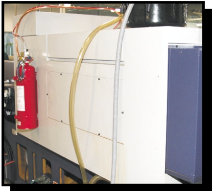
Image 2 - Installed Firetrace ILP system
