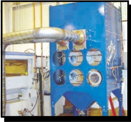
Image 1 - Full view of Dust Collector
