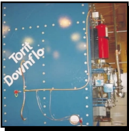
Image 3 - Installed Firetrace Indirect Low Pressure (ILP) Dry Chemical System
