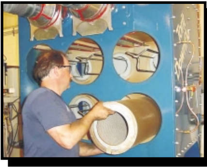
Image 2 - Filters installed on Dust Collector
