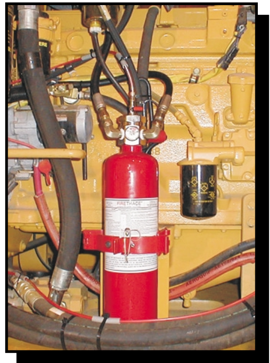
Flexible discharge lines are used.
