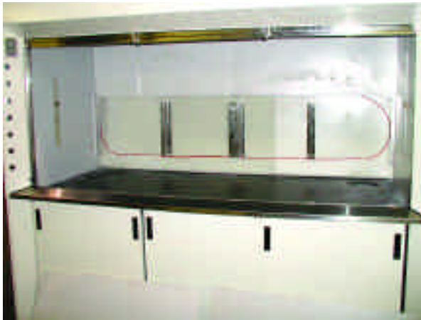
Figure 2 Firetrace detection tubing mounted across the baffles of a fume cabinet.
