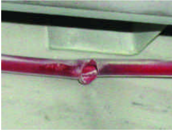
Figure 1 An actual tubing burst from a fume cabinet fire.
