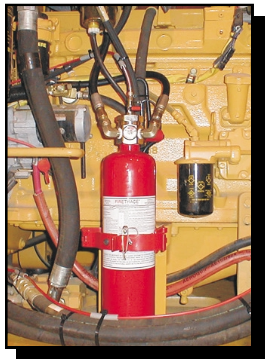
Flexible discharge lines are used.
