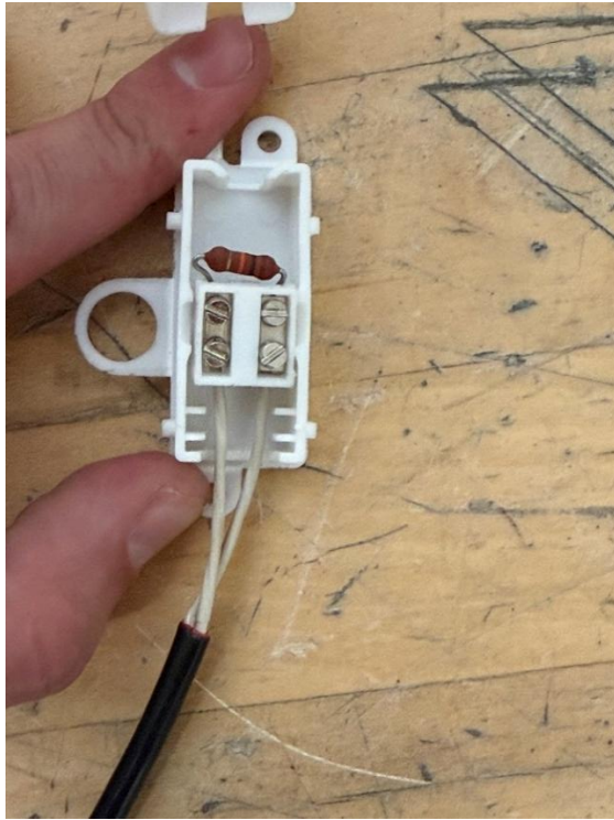
Figure 12: Linear Heat Detection End of Line Termination Box with 10kΩ Resistor
